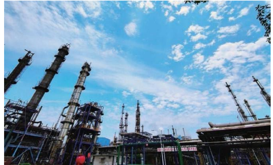
The 50 KTPA eco-friendly equipment for high-concentration methanol effluent disposal, the 35 KTPA waste sulfuric acid recycling equipment, and the equipment for drying and comprehensive utilization of carbon black constructed by Sinopec Chongqing SVW Chemical Co., Ltd. With them, the recycling of hazardous waste is available. The annual recovery of methanol is 26,000 tons, sulfuric acid is 30,000 tons, and the annual production of carbon black filter cake is decreased from 40,000 tons to 10,000 tons, which can be reused as fuel; thus, the comprehensive utilization rate of hazardous waste reached 98.9%.
