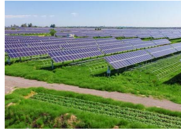
Fenglei Photovoltaic Power Station of Sinopec Star
