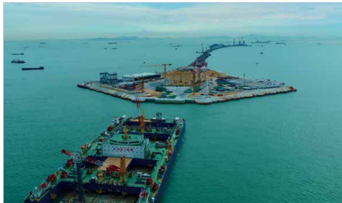
The floating installation of the first section of immersed pipe of Shenzhen-Zhongshan Bridge is completed
