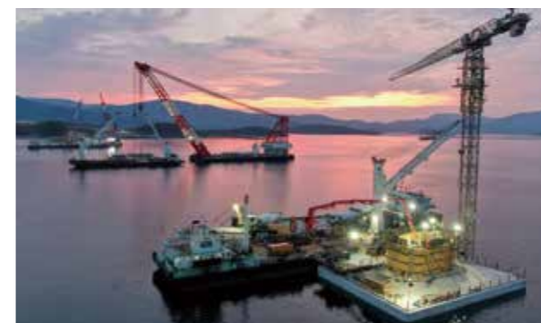
The Pelješac Bridge in Croatia is four kilometers long. In 2020, we overcame the adverse impact of COVID-19 outbreak and made steady progress in all areas of development
