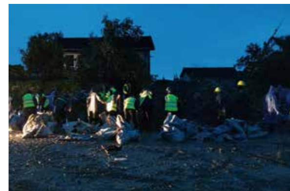
Project Department of North Extension Railway Line at Tianfu Avenue of CCCG Fourth Harbour Engineering
