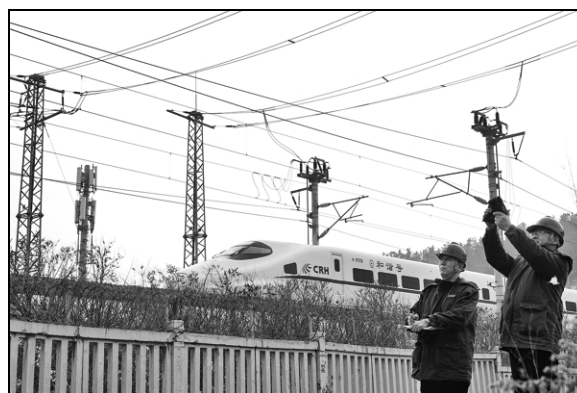
State Grid employees check railway power supply equipment in Yantai, Shandong province. TANG KE / FOR CHINA DAILY
