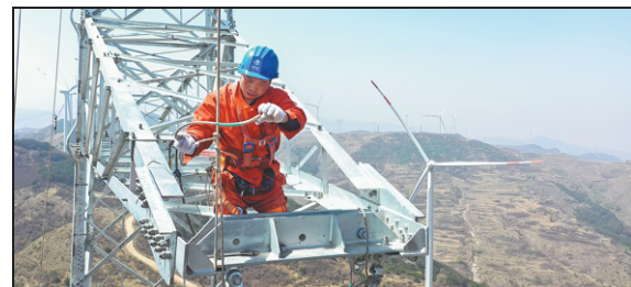
A worker installs cables on top of a pylon as part of a grid upgrading project in the city of Jinzhong. WANG HAO / FOR CHINA DAILY
