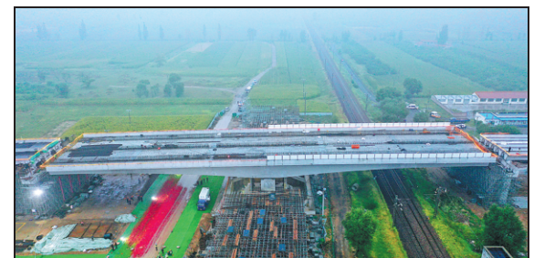
The bridge built by China Railway 15th Bureau Group is part of a highway linking Datong and Hunyuan. RUAN YANG / FOR CHINA DAILY
