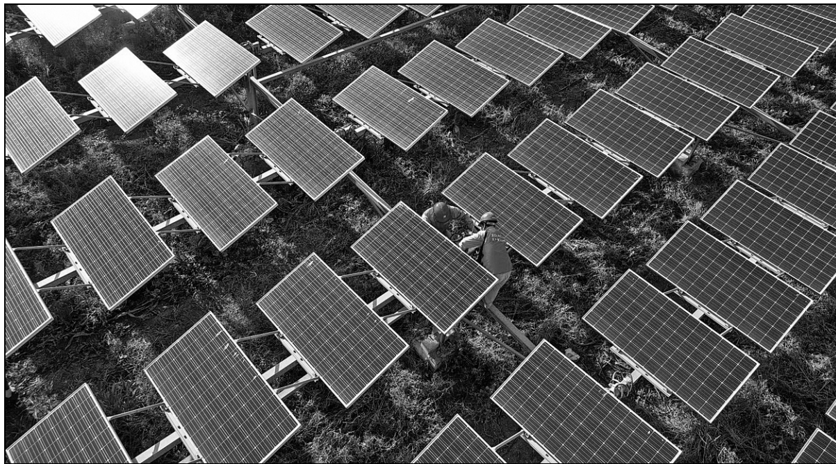
Technicians check photovoltaic panels at a solar power station in Yicheng, Hubei province, in September. WANG HU / FOR CHINA DAILY
