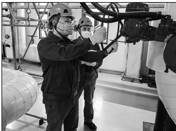
Engineers check the heating system at Shandong Nuclear Power Co in Haiyang. JIANG TAO / FOR CHINA DAILY
