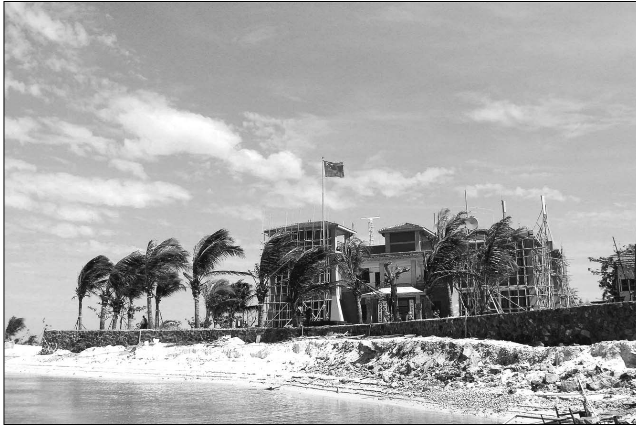
A government building under construction on Zhaoshu Island. XU WEI / CHINA DAILY
