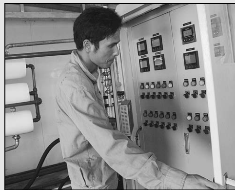
Wang Junning checks equipment at a desalination plant.
