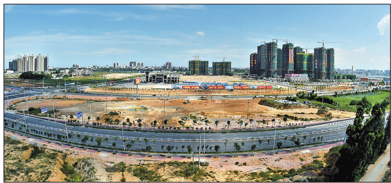
Construction of infrastructure such as roads has been stepped up in Haidong, making the zone ready to accommodate more investments from home and abroad. PROVIDED TO CHINA DAILY
