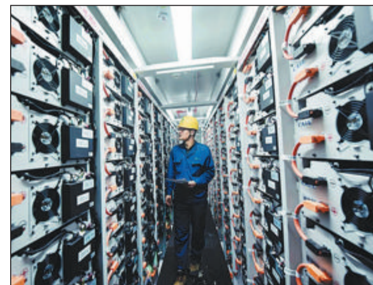
A technician inspects equipment at a power storage facility in Hangzhou, Zhejiang province, in April. LONG WEI / FOR CHINA DAILY
