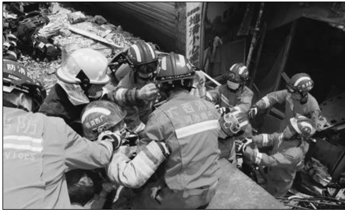
A trapped firefighter is rescued from the rubble of a market in Nandan county, Guangxi Zhuang autonomous region, on Sunday. A fire that broke out in the market at about 4:30 am was put out about three hours later. However, at 8:33 am, the market collapsed, trapping three firefighters who were investigating the site. Two were rescued, but the third, Wei Anwei, died. PROVIDED TO CHINA DAILY
