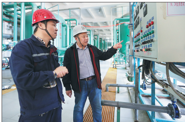
Zuo Qiwei (right), a staff member of the Administration of Work Safety in the Weifang Hi-Tech Industrial Development Zone, inspects equipment at Weifang Huawei Thermal Power Co.
